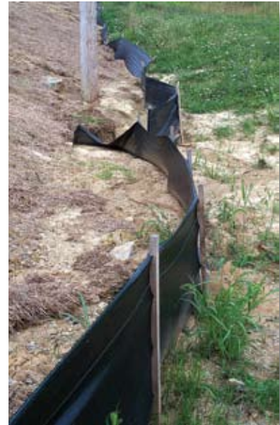
Silt fence is functioning well, but needs maintenance. Set fences back from the toe of the slope, to allow room for sediment to accumulate and maintenance.
